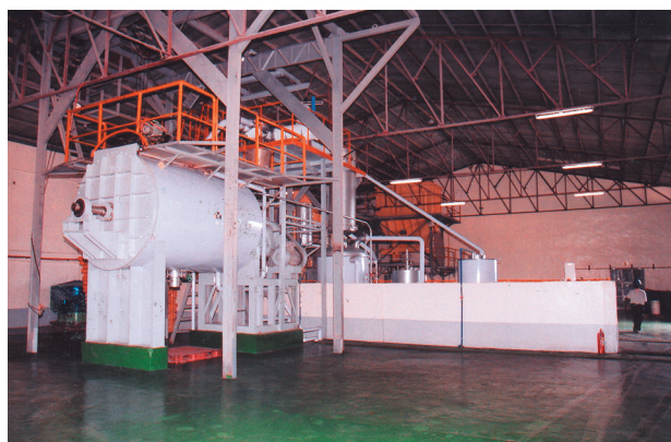
Zamboanga Carageenan Manufacturing Corporation Plant, a DBP-assisted project involved in the development of the seaweed industry.
