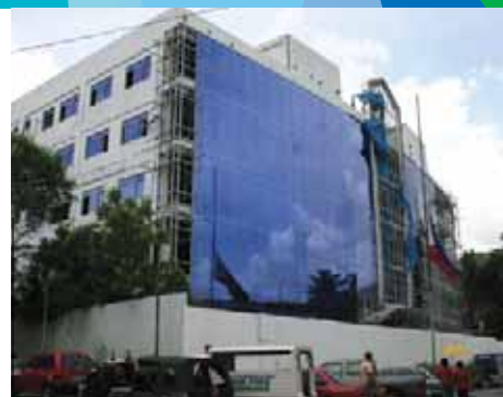
The construction of the Mandaluyong City Hall was one of the major LGU projects financed by LBP.
